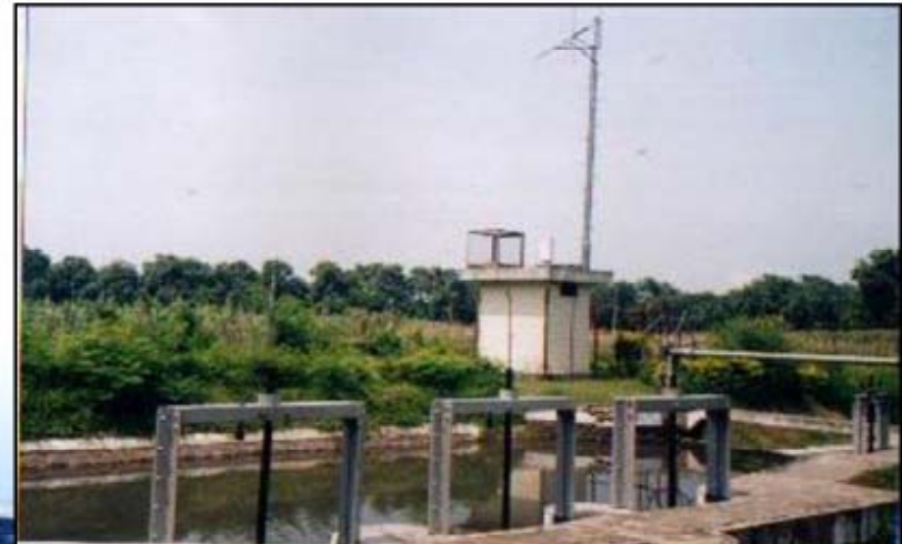
RAINFALL GAUGING STATION
